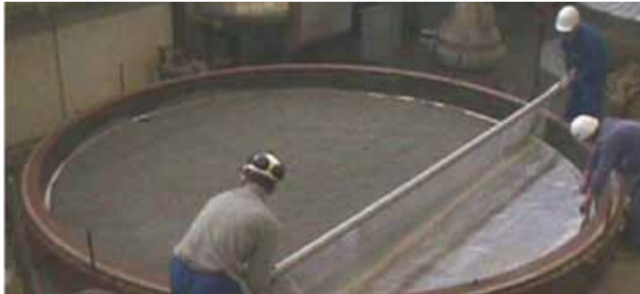
Figure 6: a. Installation of a BASF N_2O decomposition catalyst (top) b. Placing the Pt gauze over the decomposition catalyst (bottom)
